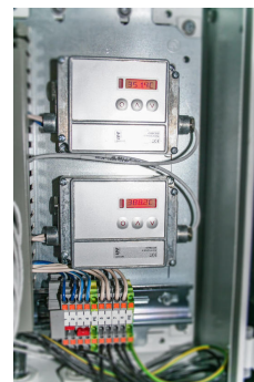
The two evaluation units are located in a thermally less critical area in a separate housing on the rotary kiln.
